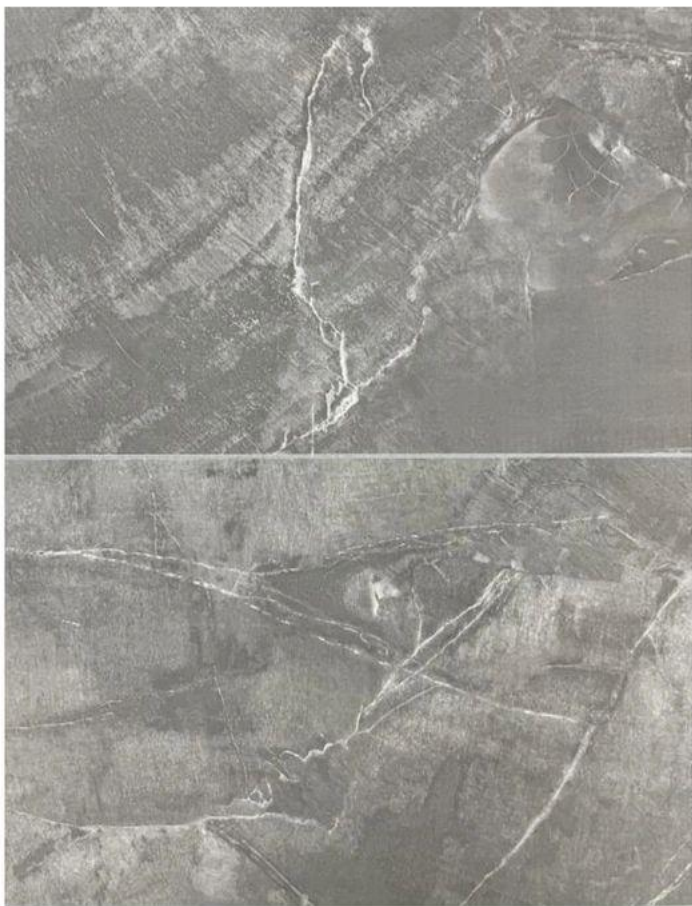
15"x26" Cracked Slate
